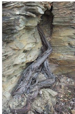
Figure 1. Thick tree root which contributed to a 4m 3 wedge failure.
